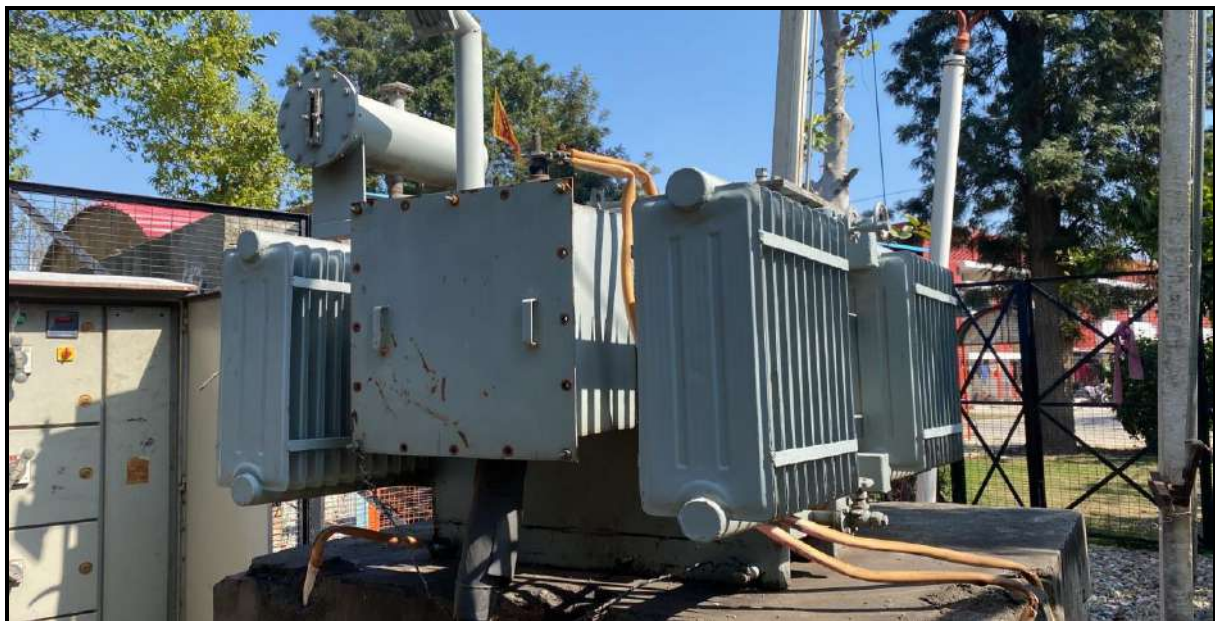
Figure: - 315 kVA Transformer near C- Type Quarter
