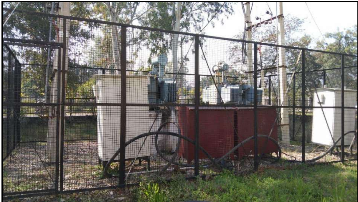
Figure :- 315 kVA and 250 kVA TRs installed Near IIE Building (Chemistry and Environment)
