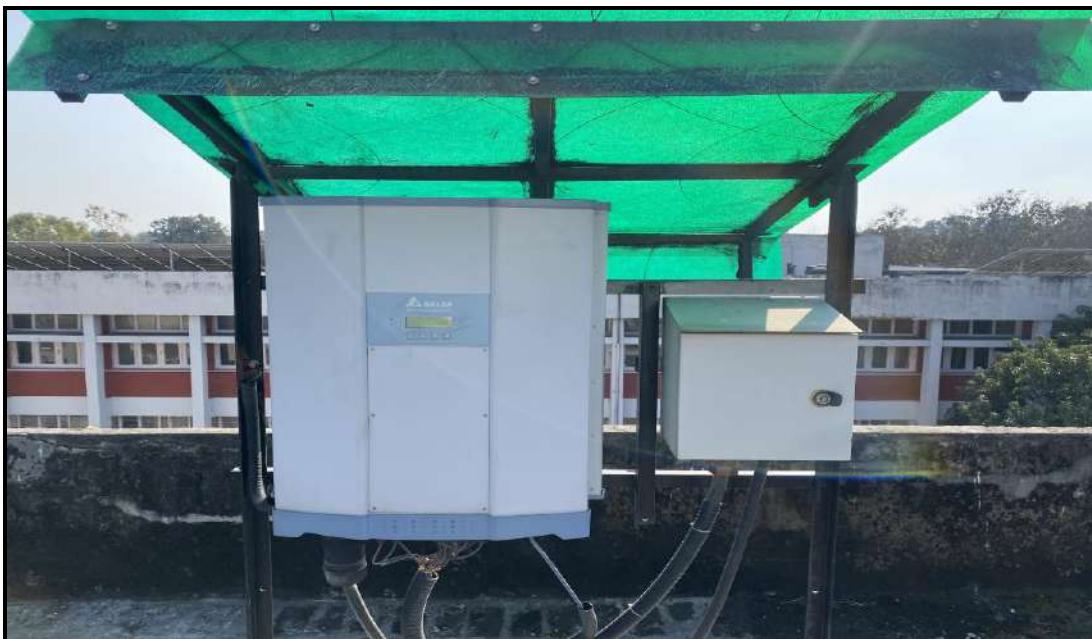
Solar Inverter at Different Buildings
