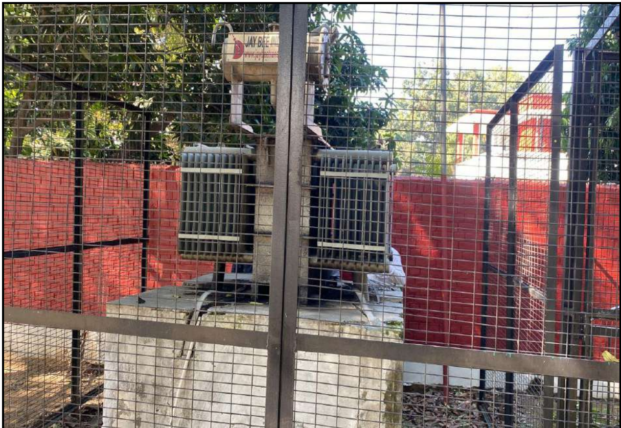
Figure :- Two 315 k transformers- one is near E-17 and second is near E-28
